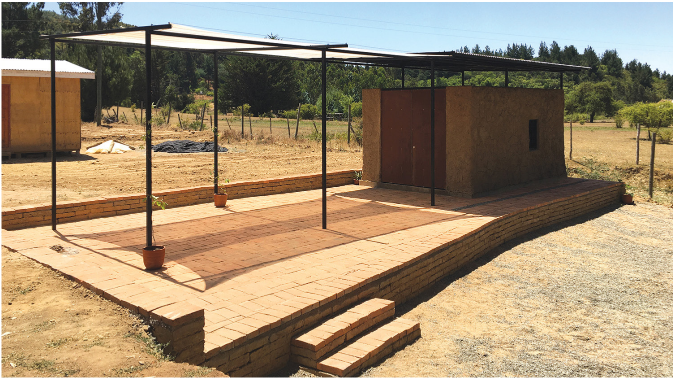
Figure 2. A new workshop and meeting place in Pílen. The plinth is constructed with fired clay bricks, while the metal structure and the workshop room are made using the “Techno-Quincha.” Ivy plants will replace the mesh at the base of the pillars to provide shade. The Authors
